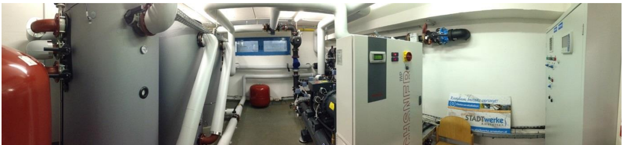
Figure 2: Heat pump of STADTwerke Amstetten using the nearby sewage as a source (right side) and three 1.5 m 3 storages (left side), source: OCHSNER Wärmepumpen GmbH
